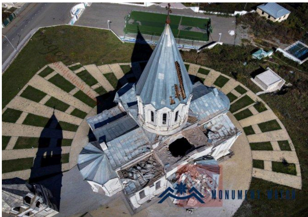
Figure 2 - Aerial view of the church after bombardment 19
